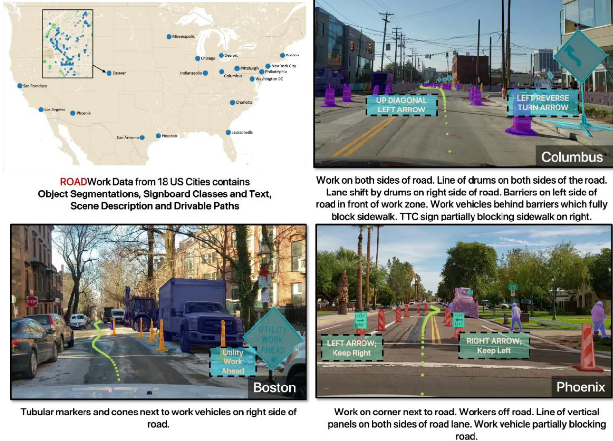
Figure 1 Overview of the ROADWork Dataset. A multi-city collection (18 US locations) featuring comprehensive annotations for autonomous navigation in work zones [1].
